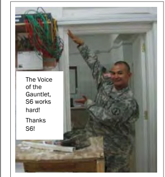
SSG Zarco, S6 NCOIC, proudly displaces switches he and his section installed. Getting the new headquarters compound wired for internet was the priority mission for the S6 section. Soldiers of the S6 worked hard to accomplish the mission in time for the battalion to assume operations.
